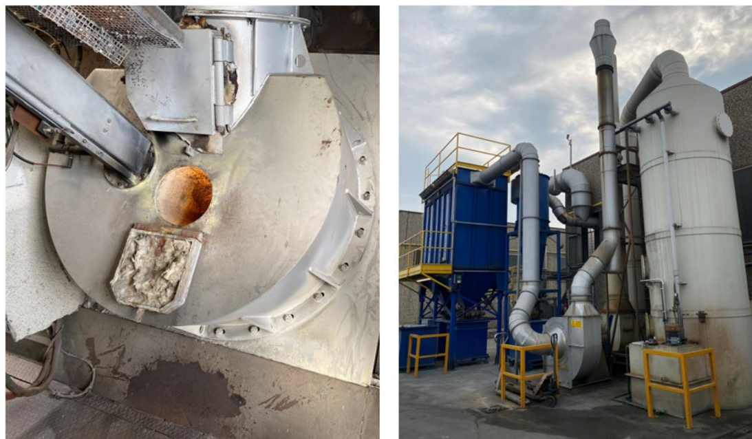
Figure 4: Feeding port and off-gas treatment system of a pyrometallurgical treatment plant for Li-ion batteries
